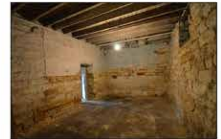
Interior view across room 1.3. Openings to be cut in exist slab to allow floor to vent. New flooring on top. (Ref. No.8 & No.10)
